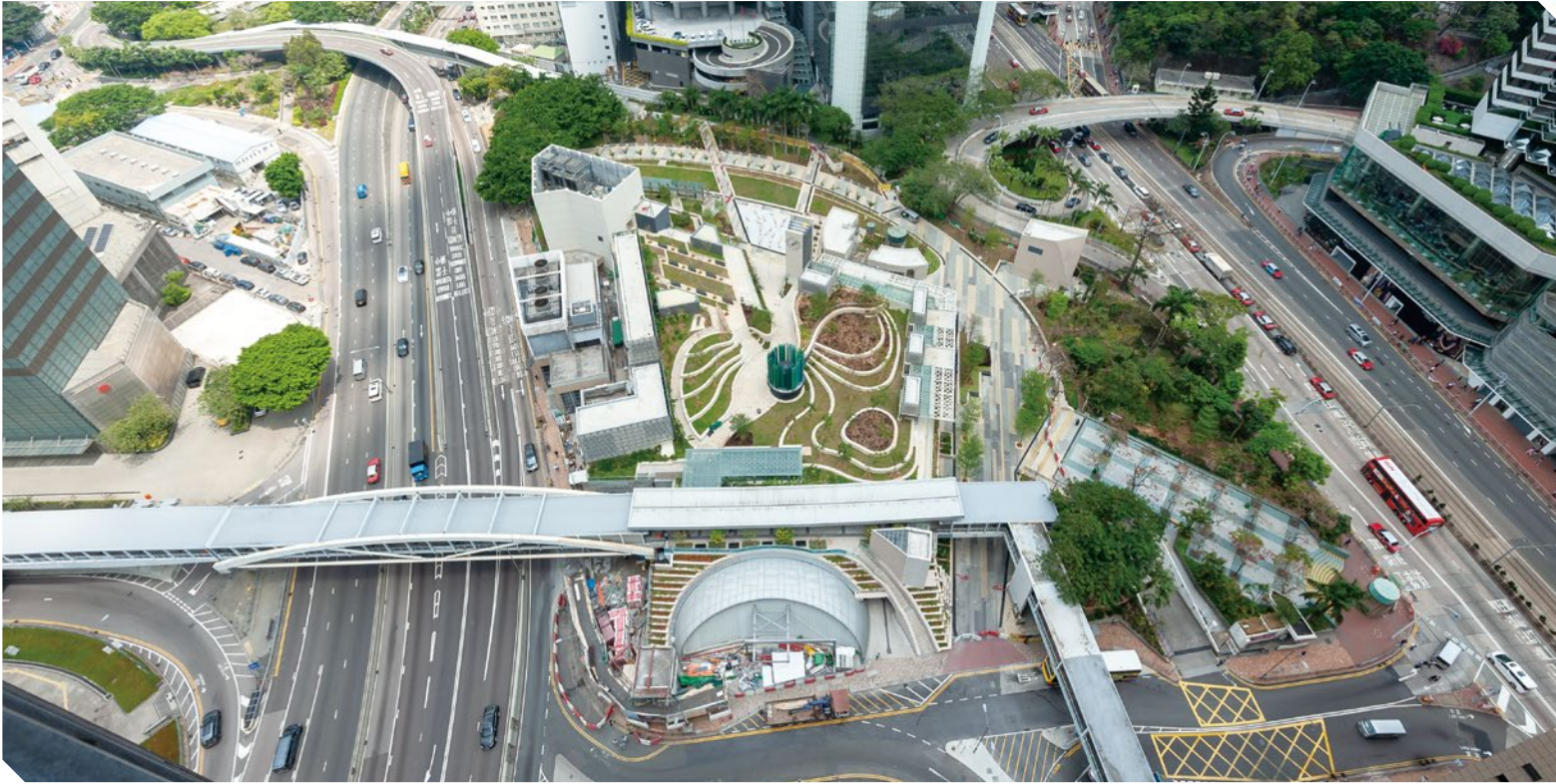
施工中的金鐘站擴展部分及重置後的夏愨花園 The expansion works at Admiralty Station and reprovisioning of Harcourt Garden
