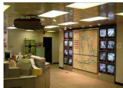
ATC Control Room
