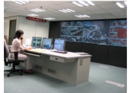
ATC Control Room
