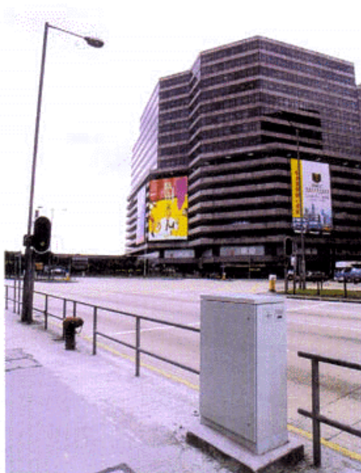
燈號控制器 Traffic signal controller
