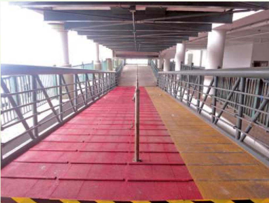
鋪有防滑物料及設有槽紋的碼頭斜道 Ramps with anti-skid gangplanks and grooves at pier
